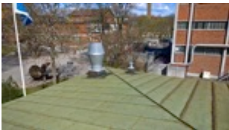
Y-2 Ventilation, utblås
