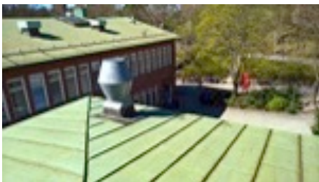
Y-1 Ventilation, utblås
